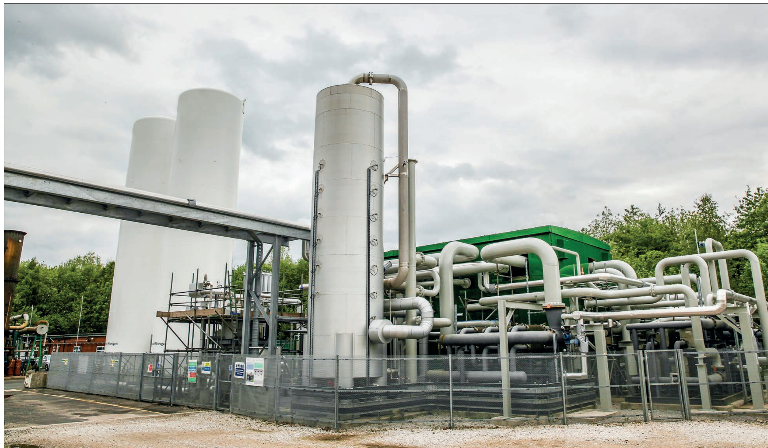
The 15MWh cryogenic energy storage demonstration plant at Bury commissioned in 2018 © Highview Power
