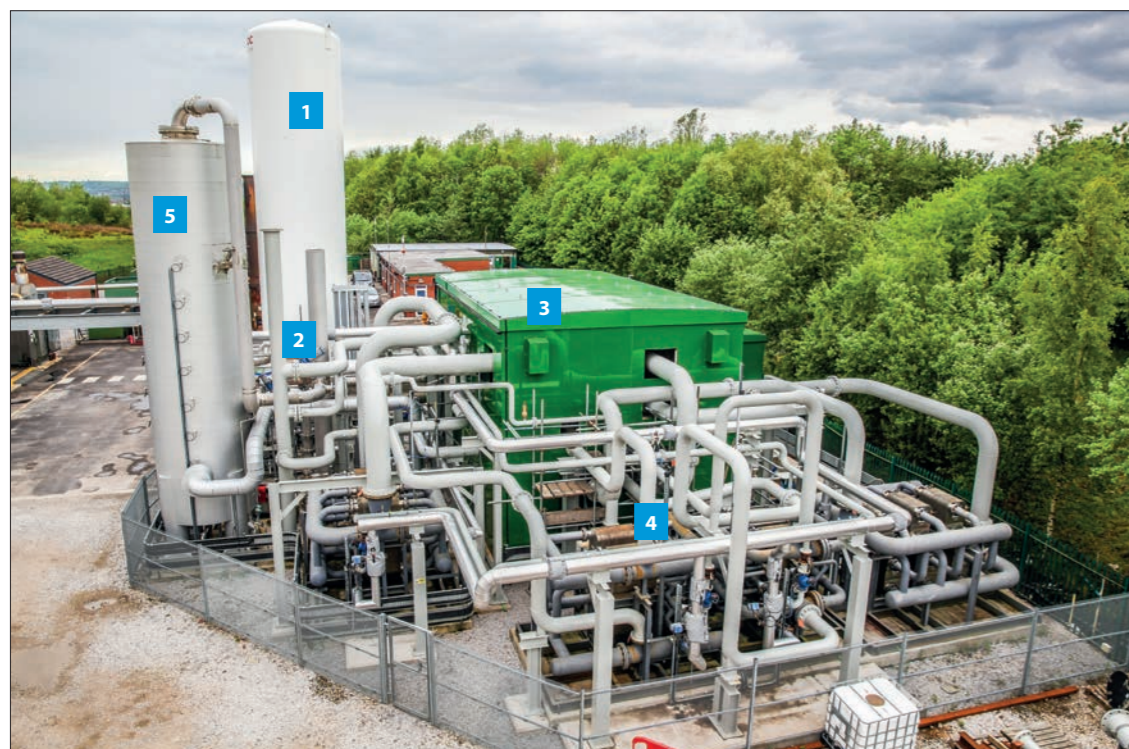
1. Liquid air storage 2. Cryo pumps 3. Containerised power turbine and generator (2 x 10 MWh) 4. Heat exchanger 5. High grade cold stores © Highview Power
